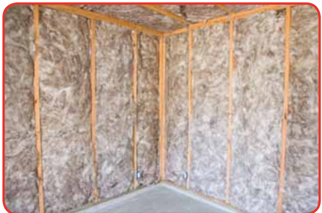
Eco friendly insulation can be put into false walls in an old home.
