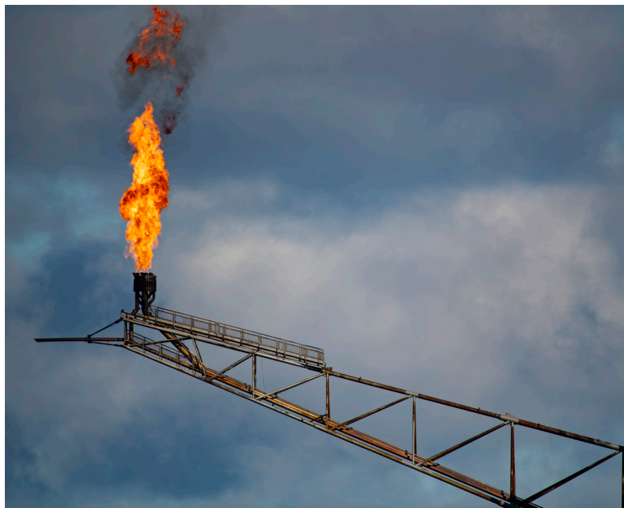
A gas flare on the Cormorant North Platform in the North Sea
